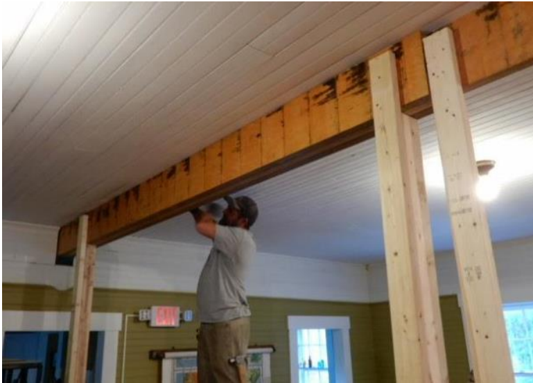
Town House Restoration: Beam installation 2 nd floor of the Town House to support the roof
