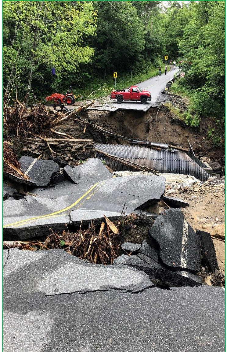
Damage from the July 2017 storm Photo Credit: The Town of Orange
