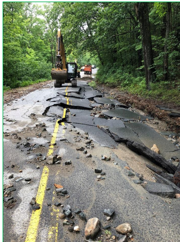
Damage from the July 2017 storm Cardigan Mountain Road Photo Credit: The Town of Orange
